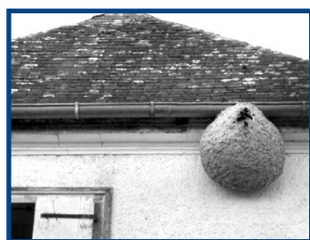
Figure 2 Asian Hornet nest under roof eave
